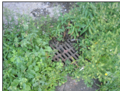
Vegetation and debris needs to be cleared from truck well drain.
