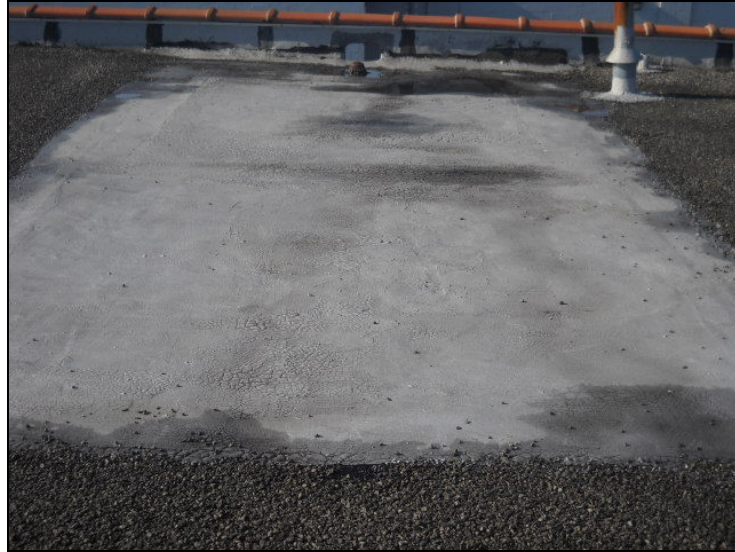
Areas of patched material.
