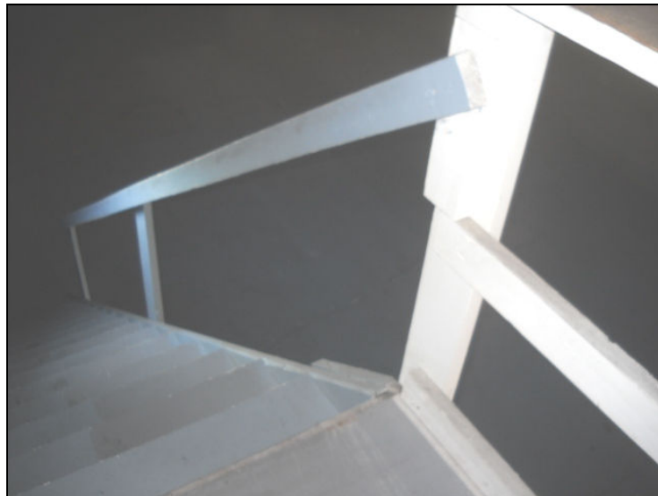
The railing construction for the warehouse staircase is improper and presents a safety risk.
