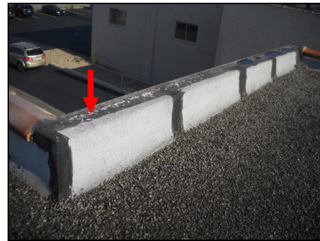
Missing coping on parapet wall.
