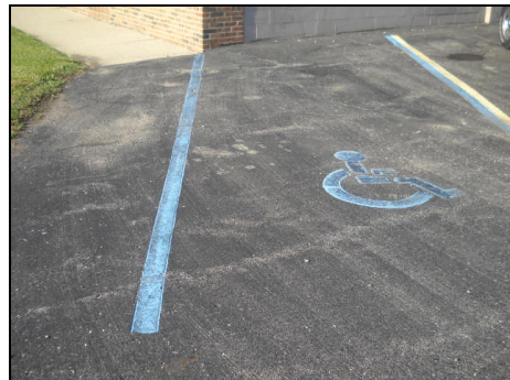
Present, yet insufficient ADA parking.
