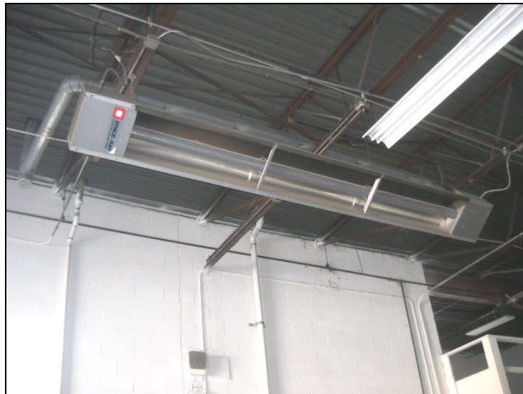
Representative view of radiant gas heater in the warehouse area.
