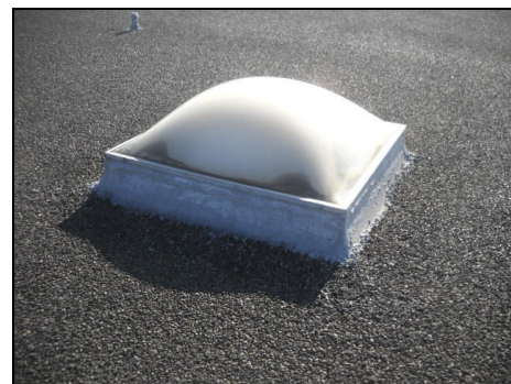
Skylight flashing needs caulking.
