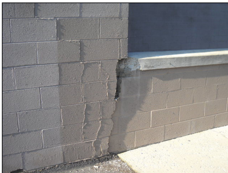
Block and cap damage at retaining wall for truck well.
