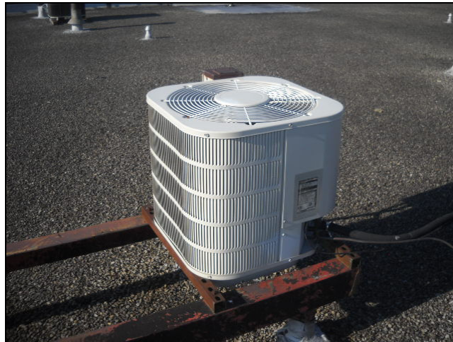
Newer condenser unit serving west side.
