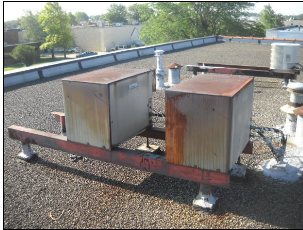
Two condenser units serving east side. These units are 20+ years old.
