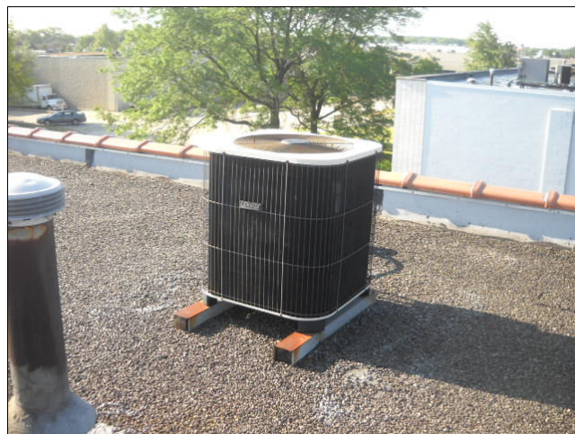
Older condenser unit serving west side.
