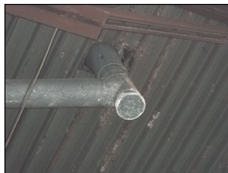
Evidence of roof leakage at chimney protrusion.
