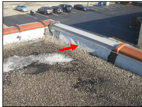
Loose material at parapet wall.
