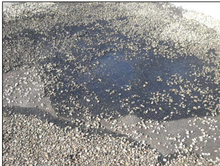
Areas of missing gravel.
