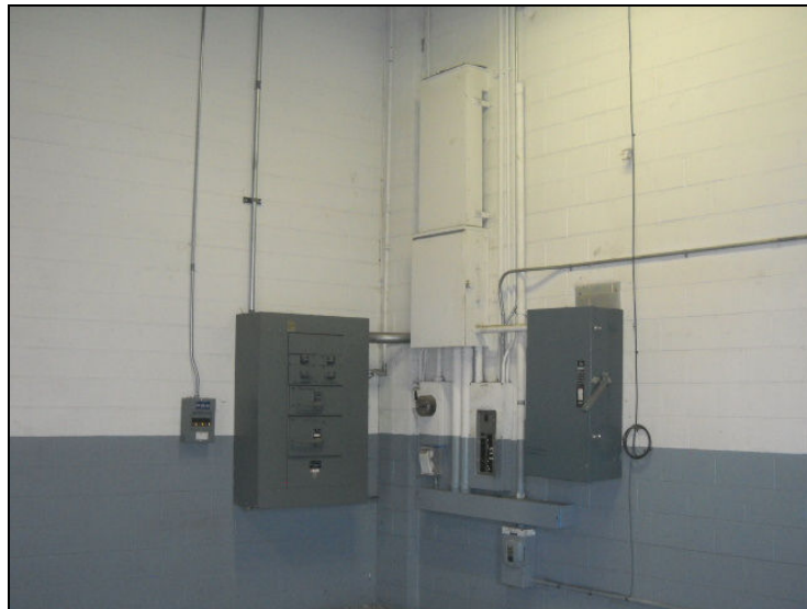
Electrical service for the north suite.
