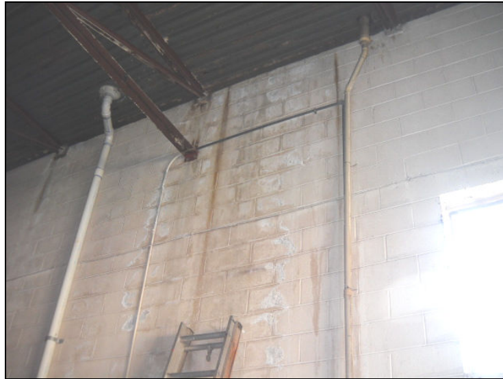
Internal water staining from roof leakage.
