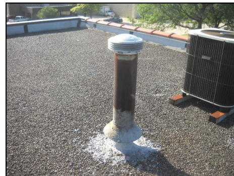
Surface corrosion on chimneys.
