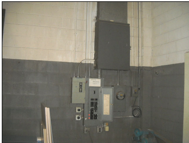
Electrical service for the north suite.
