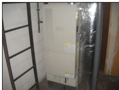
Newer furnace unit.
