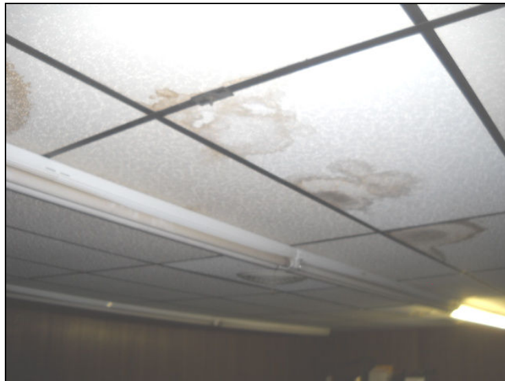
Multiple areas of ceiling tile water staining observed on 2 nd floor.
